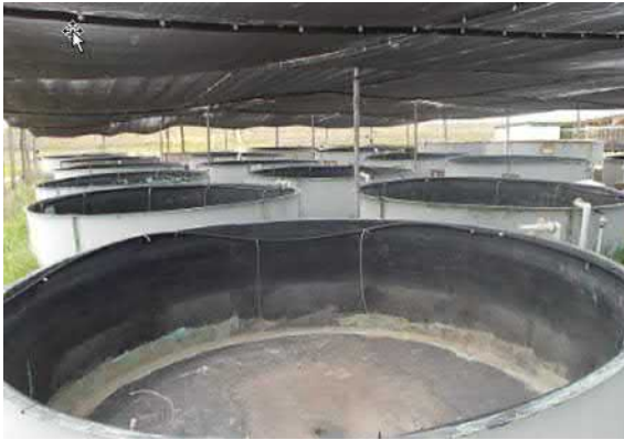
FIG. 5.3A Round fiberglass tanks used at the Texas A&M-ARML.
