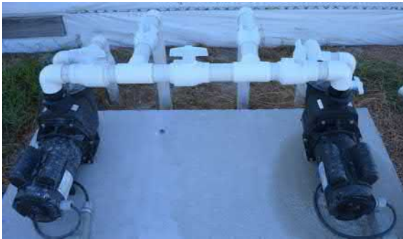
FIG. 5.38 Two 2-hp centrifugal pumps for a 100m 3 raceway. The 5-cm PVC valve manifold controls single or dual pump use. Valve handles are painted to reduce UV degradation.
