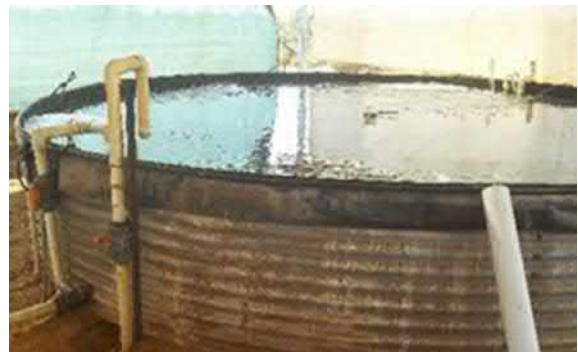
FIG. 5.3D Corrugated round tank lined with polyethylene.
